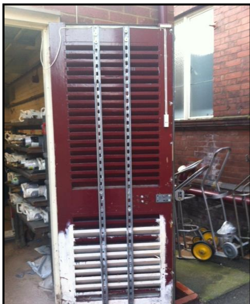
Figure 1: Metal bars have been placed to strengthen the door.
