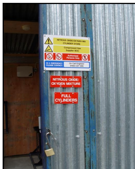
Figure 6: Poor example of securing a medical gas storage facility.
